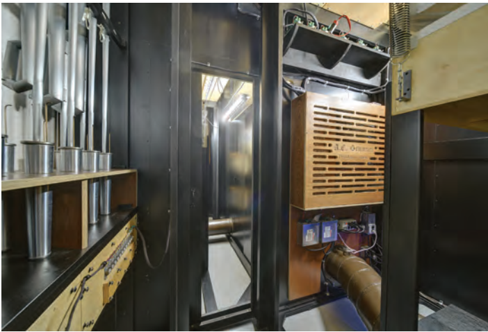
Inside the lower portion of the Swell box with the area below the Choir box beyond
