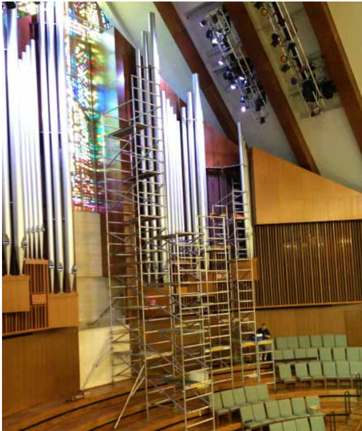
The organ facade pipe racking and structure had to be rebuilt with a significant amount of lumber and steel. Seen here is some of the scaffolding used to work on the 32' Violone pipes. (Photo credit: Brian Oliver)
