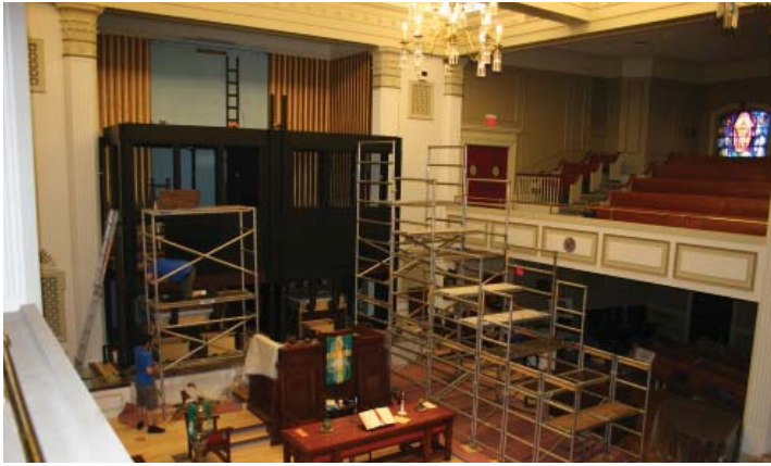
Scaffolding is erected for hoisting windchests and reservoirs to the Great and Pedal divisions on the upper level (photo credit: Jim Wilmer)
